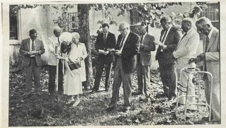
In the groundbreaking service for the addition to the Gulfview United Methodist Church gathered around pastor Si Mathison (holding bible) are: l-r, Mr. Brannon; Mr. Pinson, Mrs. Jones, Mr. Redding, Mr. Bozarth, Mrs. Eck, Mr. Prestigiacomo, Mr. Bowen and Mr. Grice.
